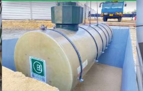
UNDERGROUND STORAGE OIL TANK
