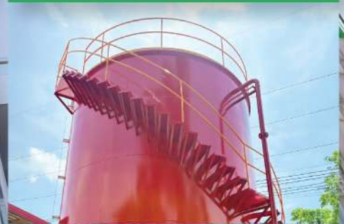
ABOVEGROUND WATER TANK
