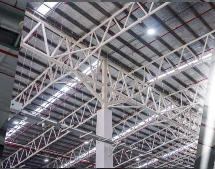
Structural Steel Truss
