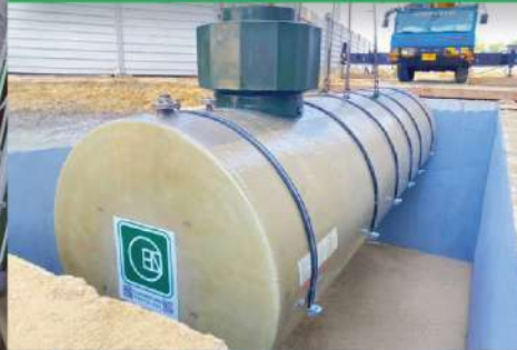
UNDERGROUND STORAGE OIL TANK
